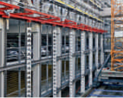
HD 200 Heavy-Duty Props as a space-saving solution: 8 m high props transfer the loads from a working and safety scaffold in a confined area.
