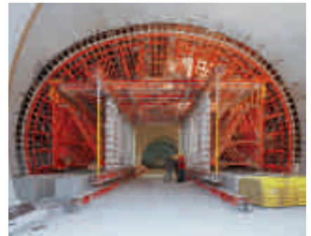
The moveable longitudinal truss – taken from the HD 200 heavy-duty system – for this tunnel was designed as a portal. This allowed a continuous flow of site traffic at all times.
