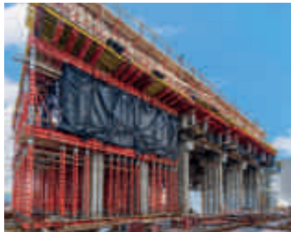
HD 200 Heavy-Duty Props as a full-surface shoring structure. The HD 200 sections were joined together, also at great heights, in order to safely transfer the loads of the 3.20 m thick reinforced concrete slab for the generator.
