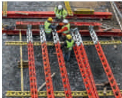
The main beam area is normally assembled horizontally – complete with diagonal bracing, working platform and access ladder.
